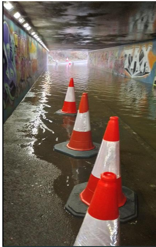
Flooding in A1(M) subway January 2023
