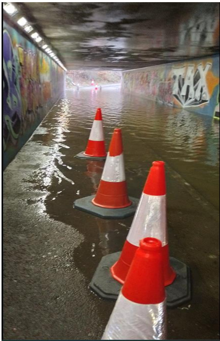
A1(M) flooding January 2023
