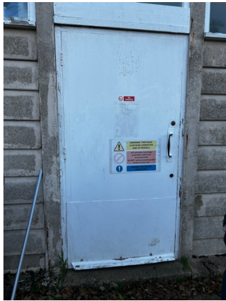
Front door with warning signs regarding asbestos
