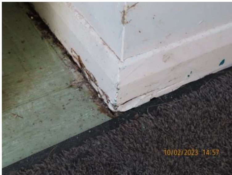
Decay on skirting near entrance door.
