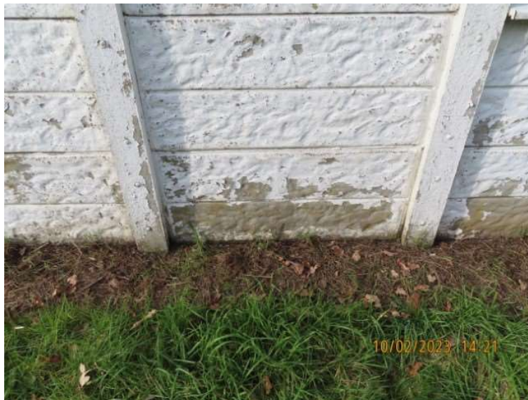
Flaking paintwork to front elevation.
