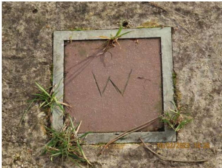
Stop valve position for water main.
