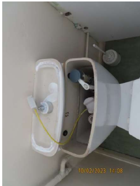
Broken flushing cistern to female WC.
