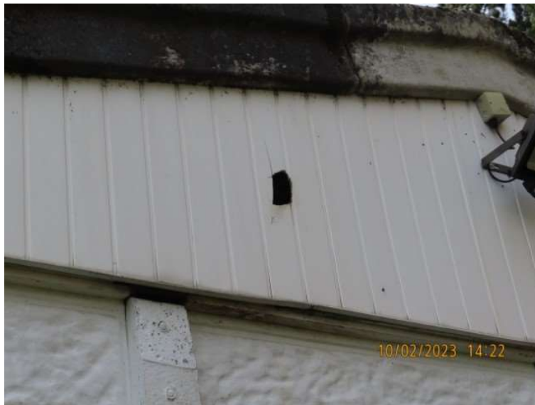
Hole in PVC weatherboarding to gable.
