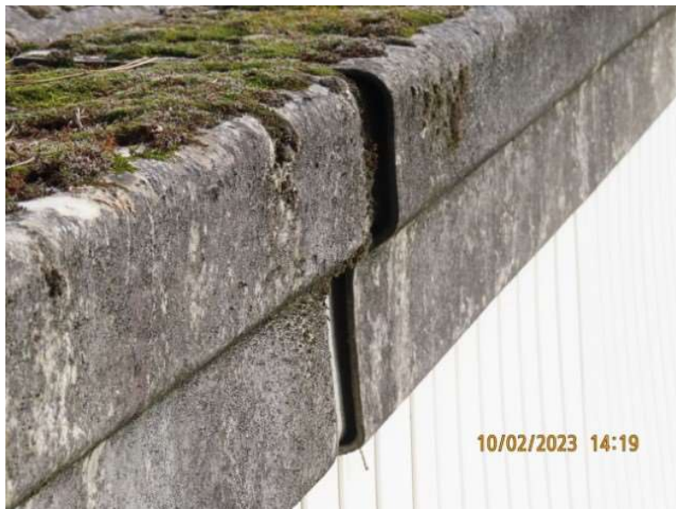
Open joint to verge capping.
