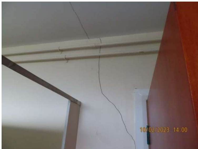
Shrinkage cracking in plaster which requires decorative repair.
