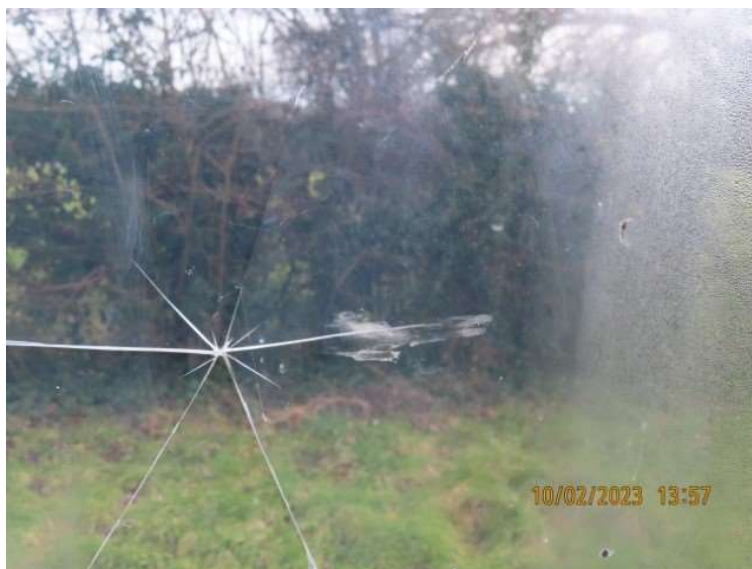
Impact damage on perspex glazing.
