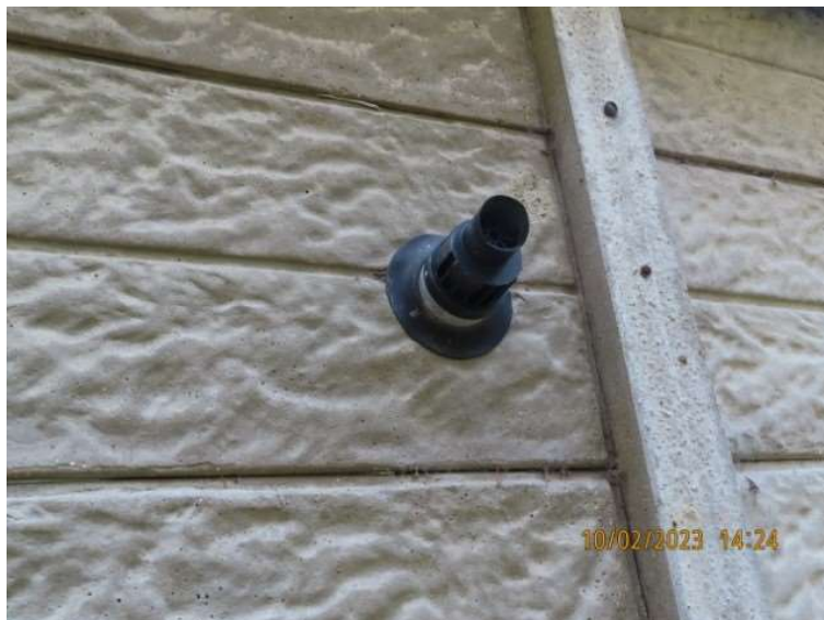
New boiler flue termination.
