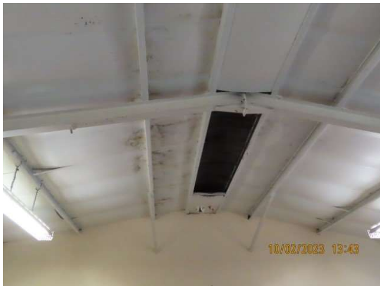
Water damaged ceiling boards through condensation staining and missing ceiling panel to ridge.
