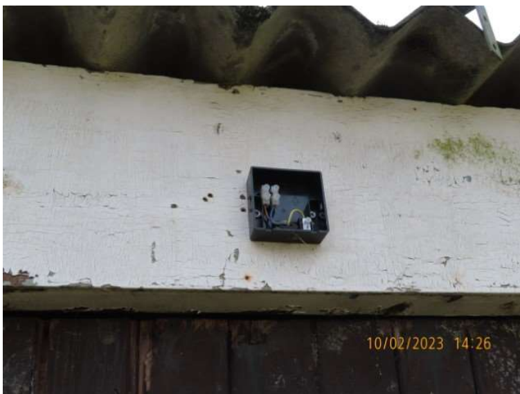
Exposed connector box with exposed wiring to garage.
