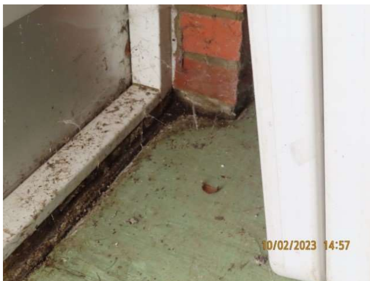
Damp flooring on entrance door threshold.
