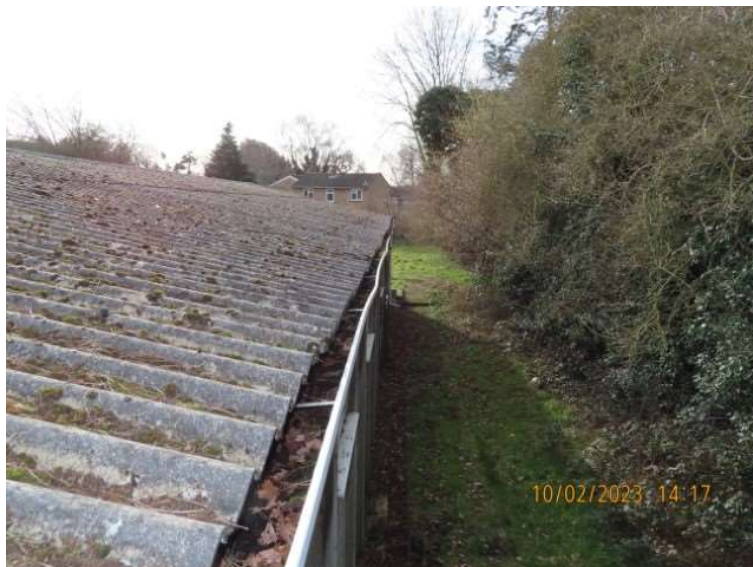
Irregular guttering to rear elevation.
