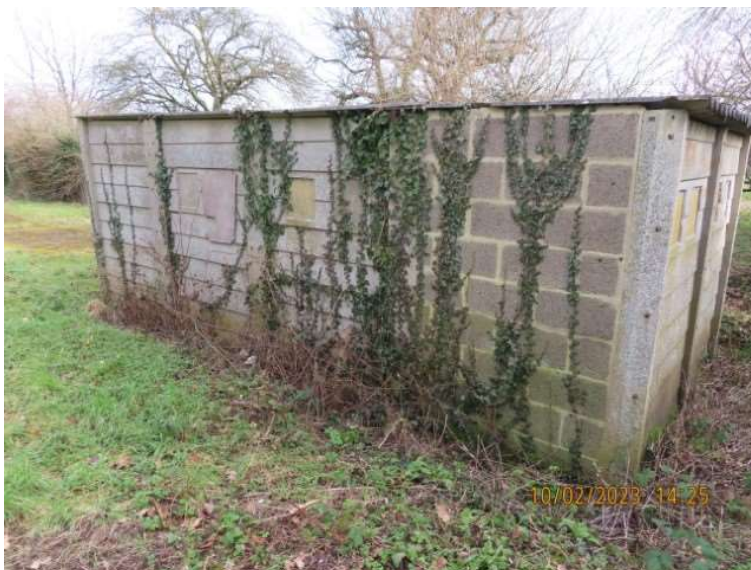
Overgrown vegetation to garage, displaced verge and broken sheets.
