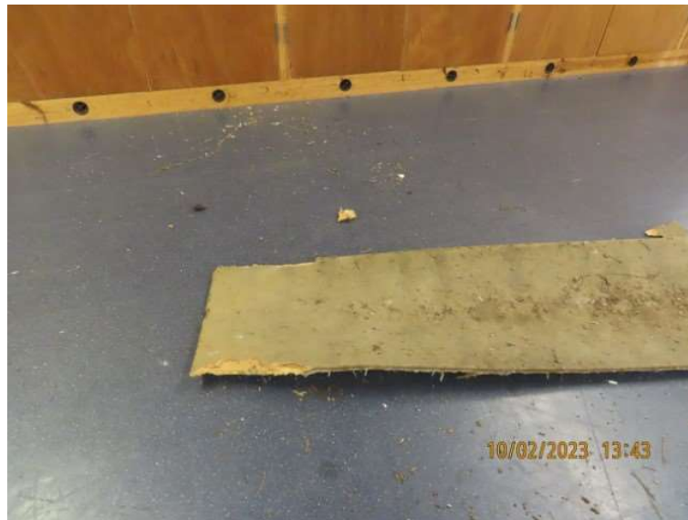
Ceiling panel fallen onto floor.
