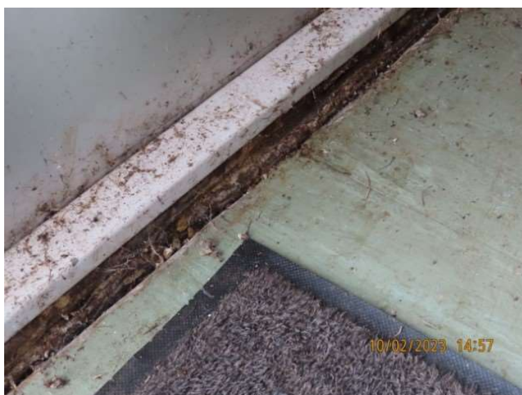
Damp flooring on entrance door threshold.
