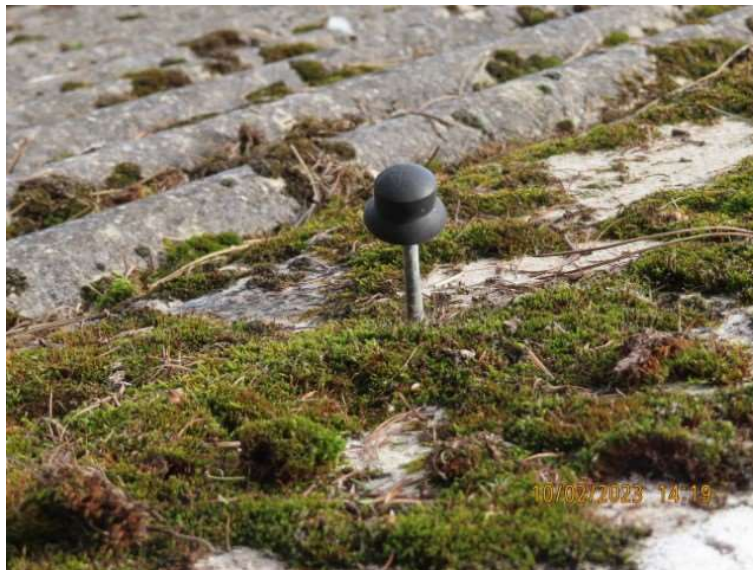
Loose fixing bolt to roof sheet.
