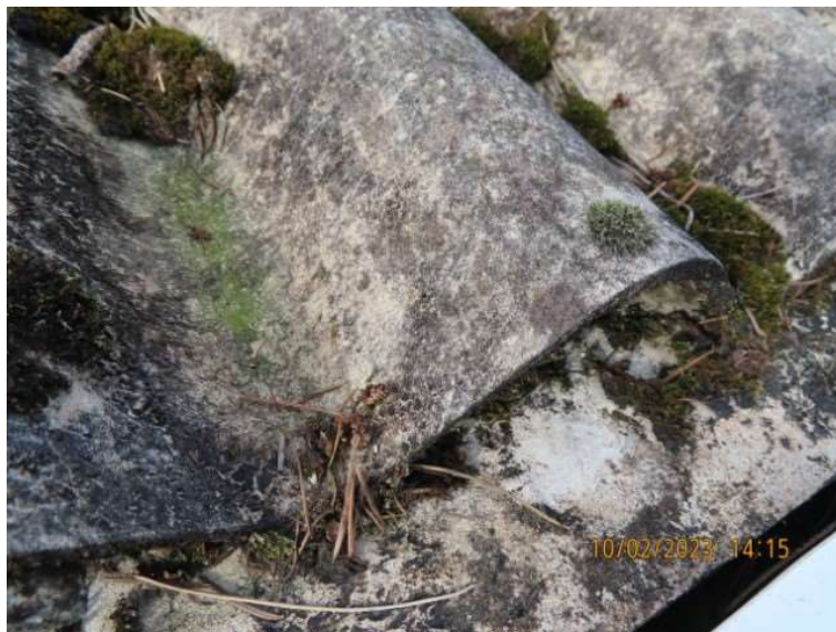
Surface degradation on asbestos cement sheeting showing signs of aging.
