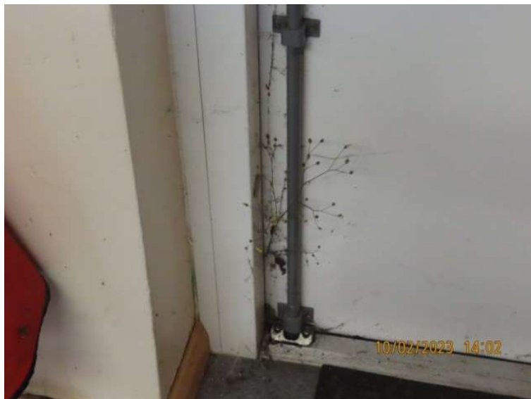
Vegetation growing through fire escape door. Note: corrosion on frame at junction with plaster.
