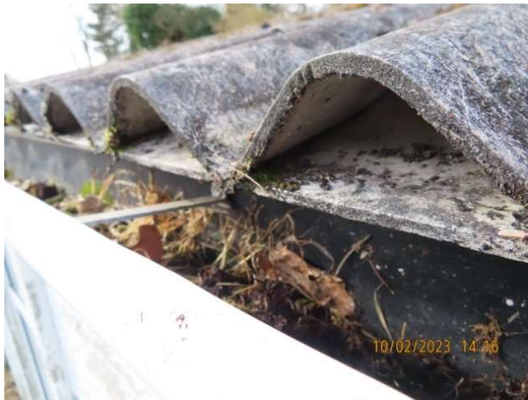
Filler pieces missing under corrugations to asbestos cement roof.
