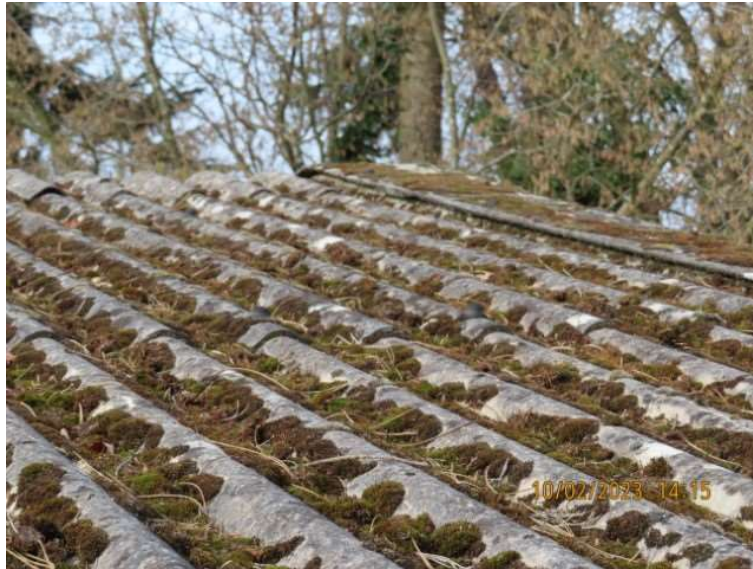
Moss growth on roof – typical example.
