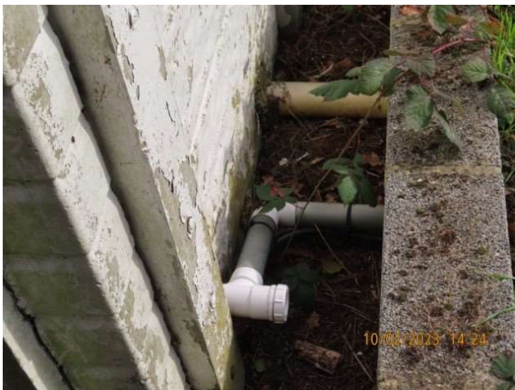
Exposed soil and waste pipe outlets to drainage chamber.
