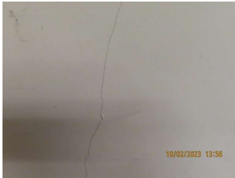
Typical shrinkage cracking in plaster wall to hall.
