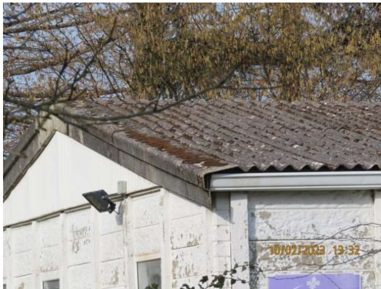
Displaced verge capping and moss on roof.
