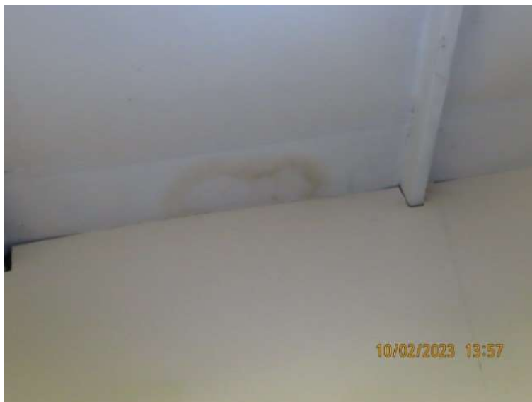
Typical water damage on hall roof.
