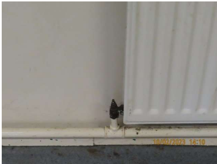
Lockshield valve cap missing to radiator – typical example.
