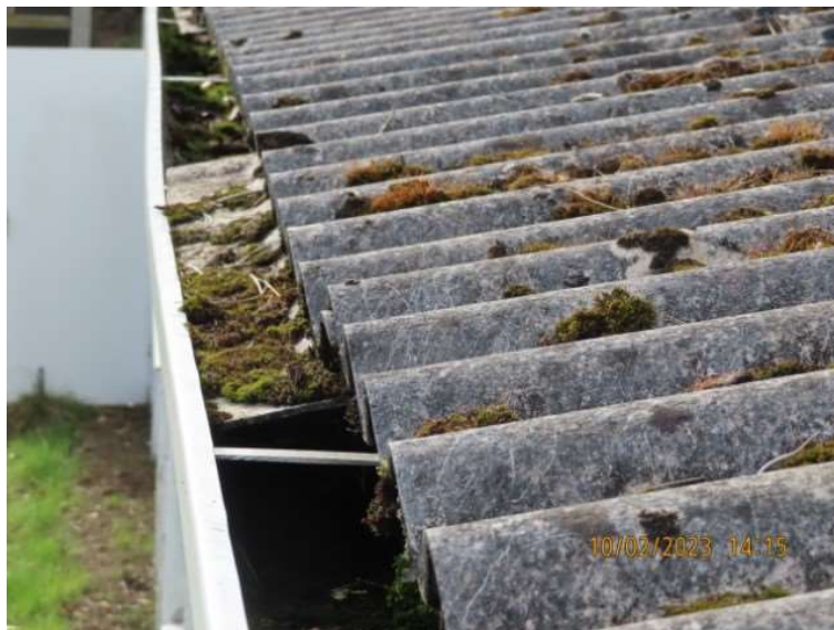
Bowing gutter and debris in gutter and moss growth on roof.
