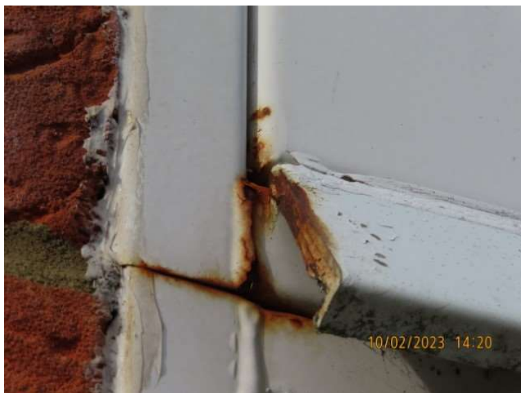
Displaced and corroded head trim to entrance door.
