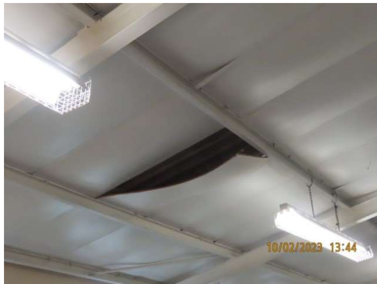
Bowing ceiling panel caused by condensation damage.
