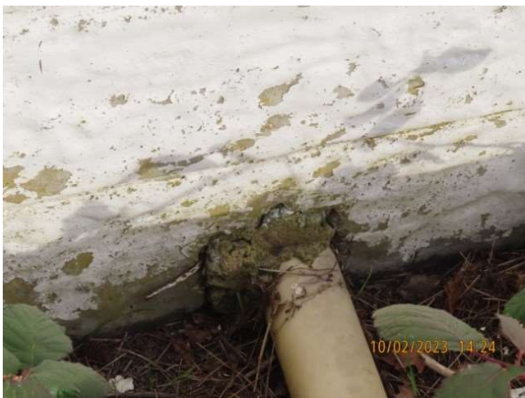
Crude infilling around soil pipe.
