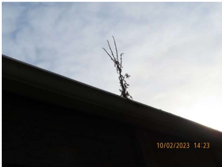
Vegetation in gutter.
