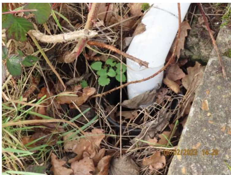
Un-sealed gulley connection to rainwater downpipe.
